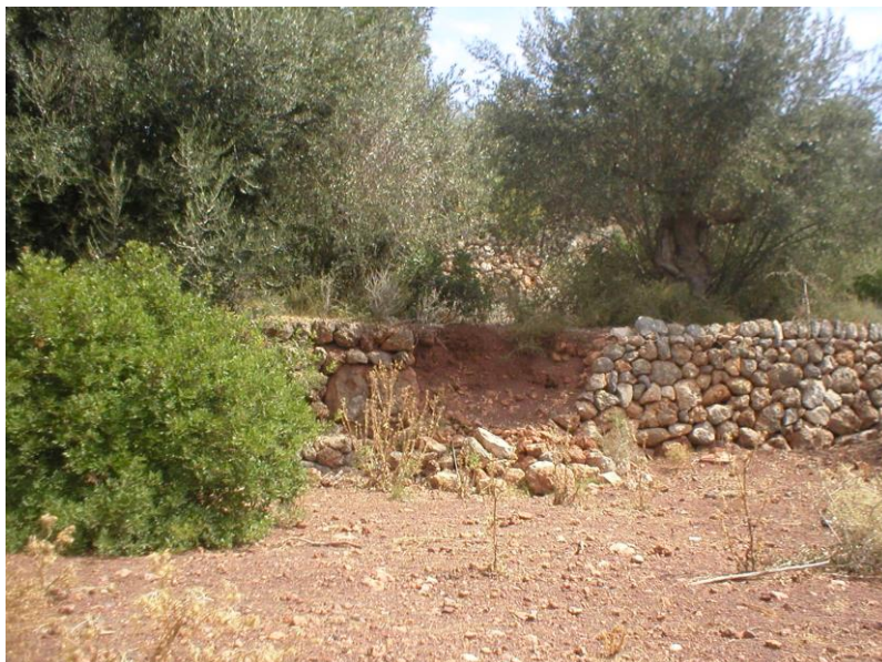
Figure 8. Wall collapsed ( Son Blanco ). Example of spoon hit collapse.
