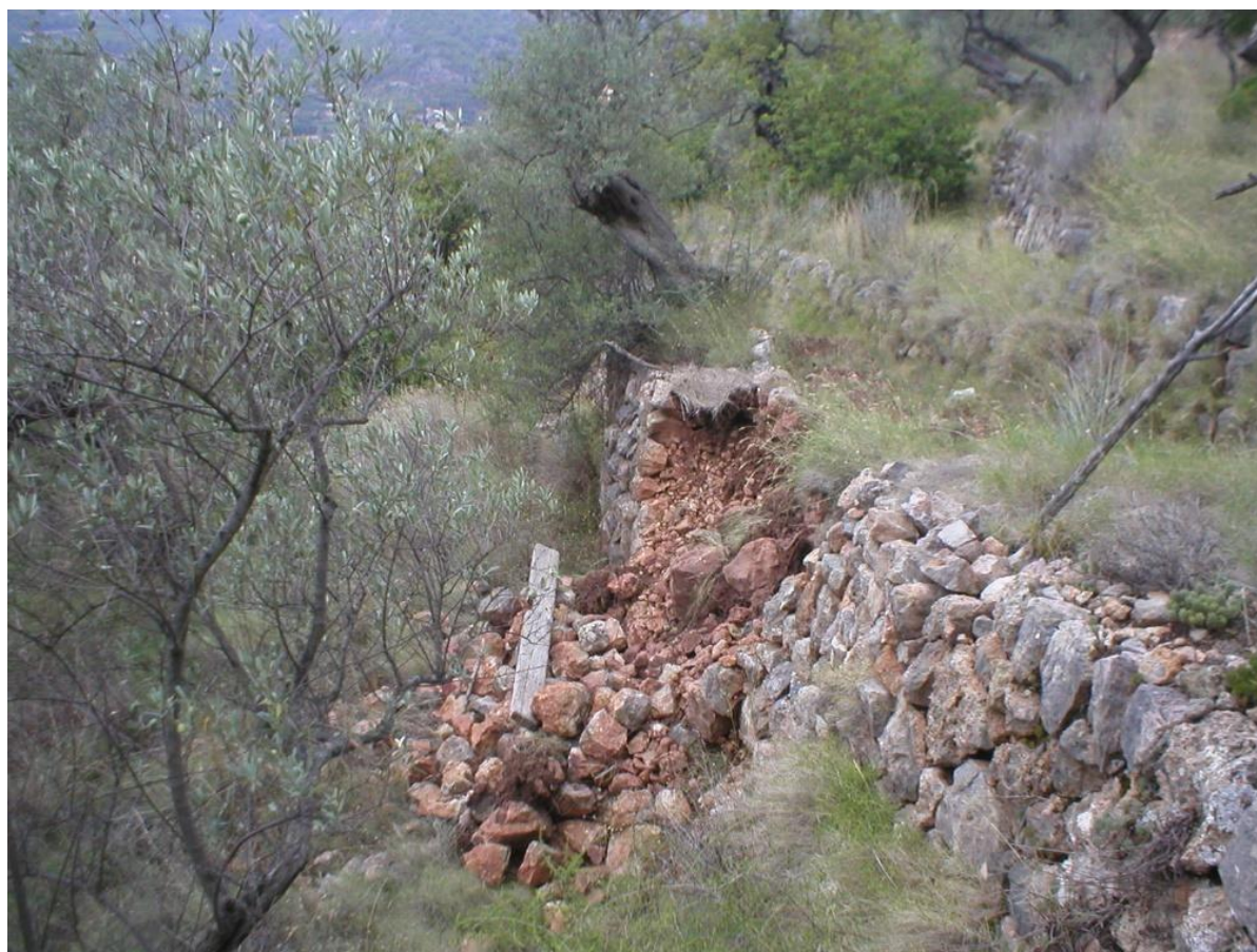
Figure 7. Collapsed wall in Ca'n Costurer plot.
